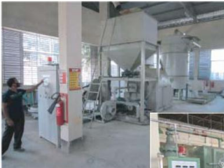
View : New Automatic Oxide Mill
